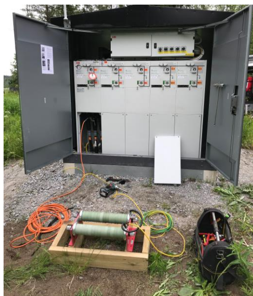
Figure 53. Primary earth fault test arrangements.
